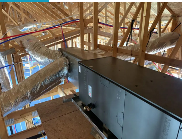
Above: Ducted Heat Pump
